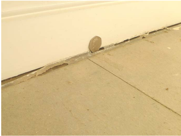
Figure 6: Failure of mastic seals due to accelerated drying during test.
