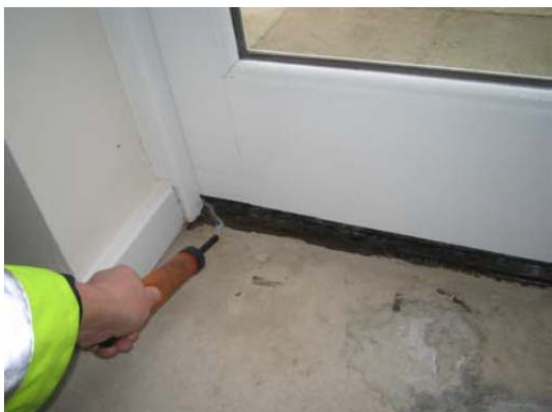
Figure 4: Air leakage under patio doors.
