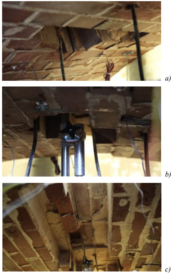
Fig. 7. Lost bricks at: a) state 1, b) state 2, and c) state 3 and 4.
